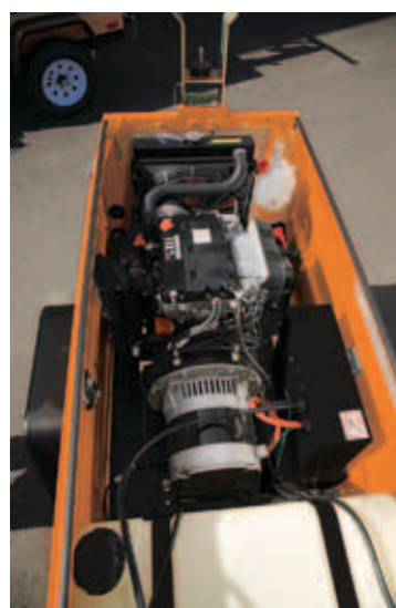
Engine access with maintenance panel open
